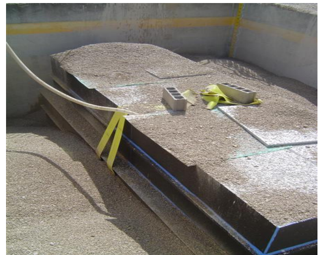
Filling the test pit with gravel and simultaneously filling the plant with water
