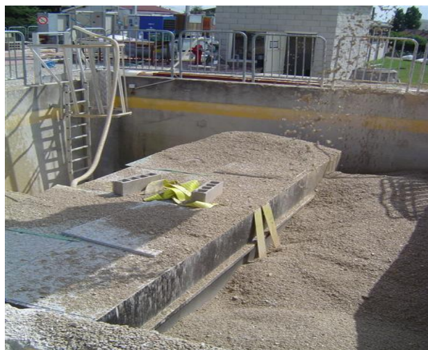
Backfilling with gravel to include the maximum backfill authorised and the pedestrian loads
